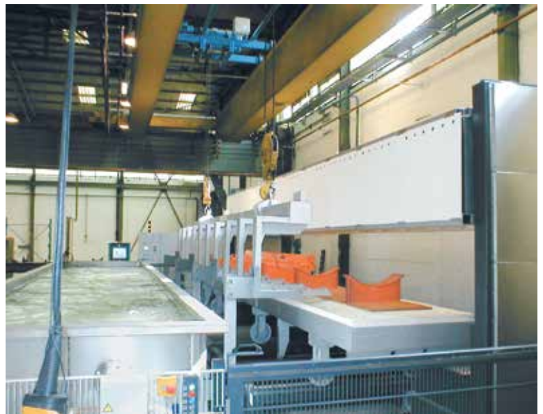
Manual tempering plant for hardening of steel rods see page 74/75
